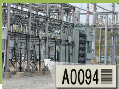
Sub Station Component Marking
